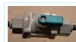
Emergency water shut-off
