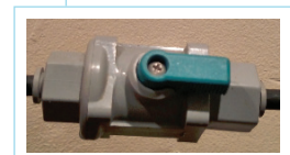
Emergency water shut-off
