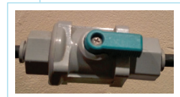
Emergency water shut-off
